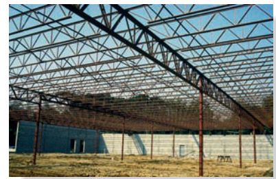
Typical interior steel pipe columns used to support the roof of a single story building.
