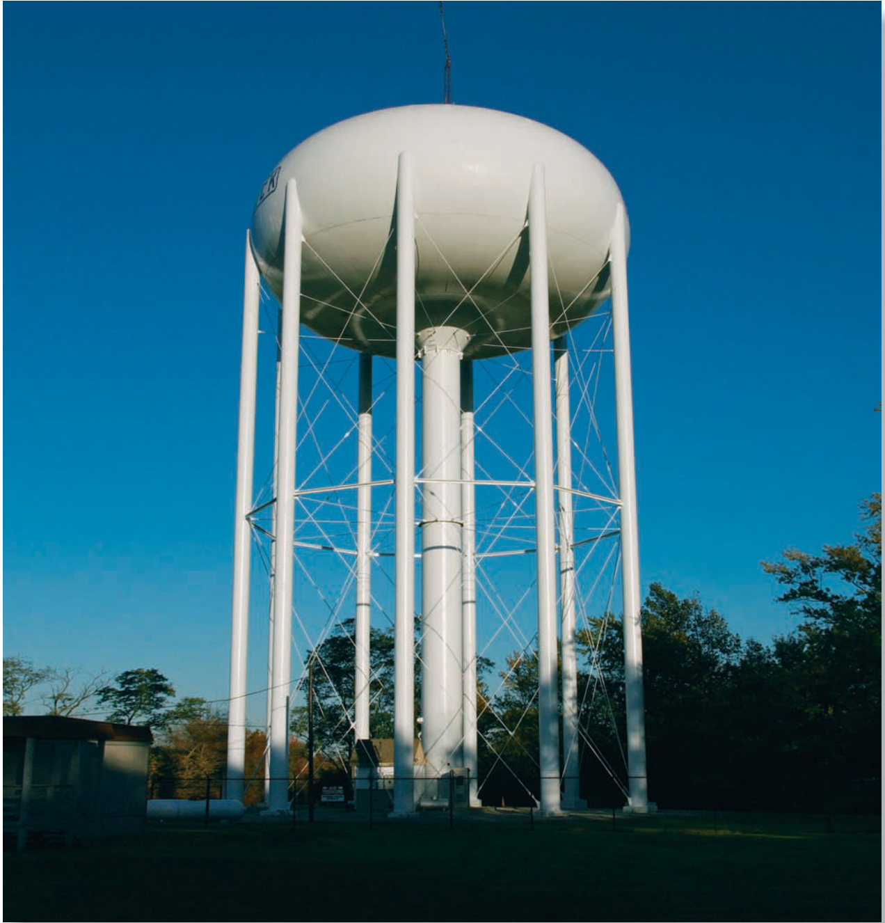
The columns used to support this water tank are braced at their mid-height in order to reduce their chance of buckling.
