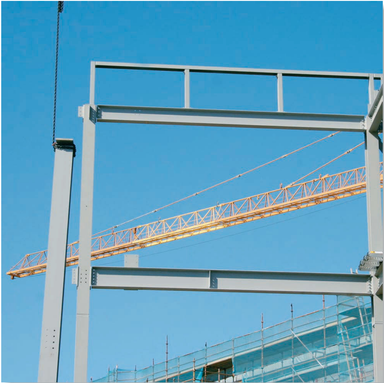
Beams are important structural members that are used to support roof and floor loadings.
